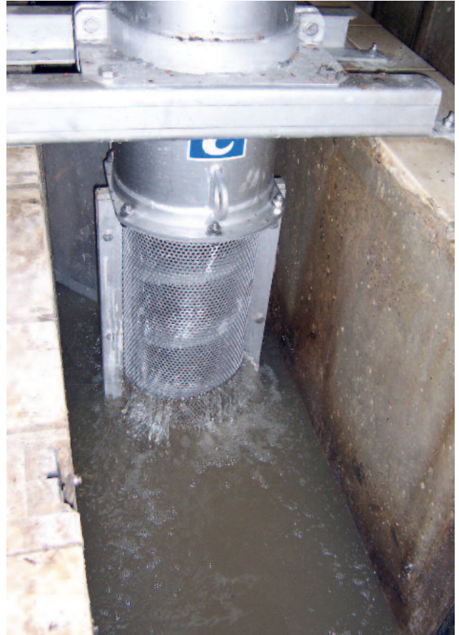
HUBER Pumping Stations Screen ROTAMAT® RoK4 in operation in the inlet channel of a WWTP
