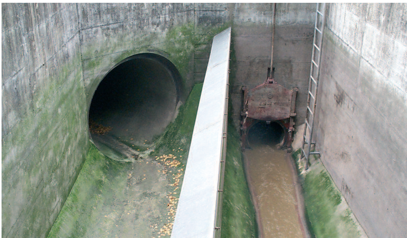
Sewers without equipment for discharge volume measurement
