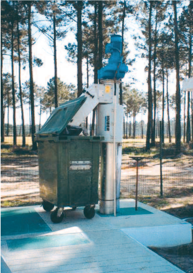
Above-ground disposal of the dewatered screenings from a HUBER Pumping Stations Screen ROTAMAT® RoK4
