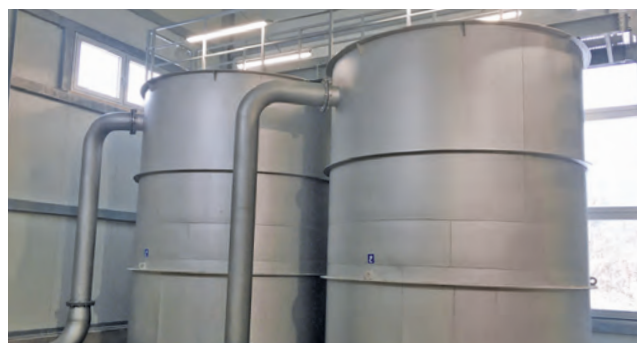
HUBER Active Carbon Filter CONTIFLOW® GAK for removal of trace substances on a municipal sewage treatment plant.
